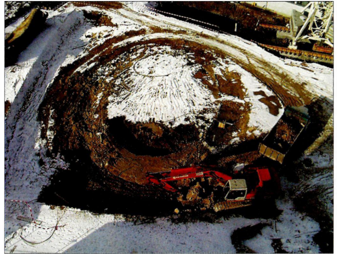
Excavation work begins at the far end of CERN's Meyrin site for the access shaft for one of the two transfer tunnels which will take protons from the SPS to the LHC. During LHC construction the big LHC magnets will be lowered down this shaft.
