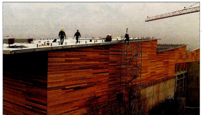
Across the road from CERN's main entrance, work advances on the large building which will shelter the shafts down to the large underground experimental area for the ATLAS detector.
